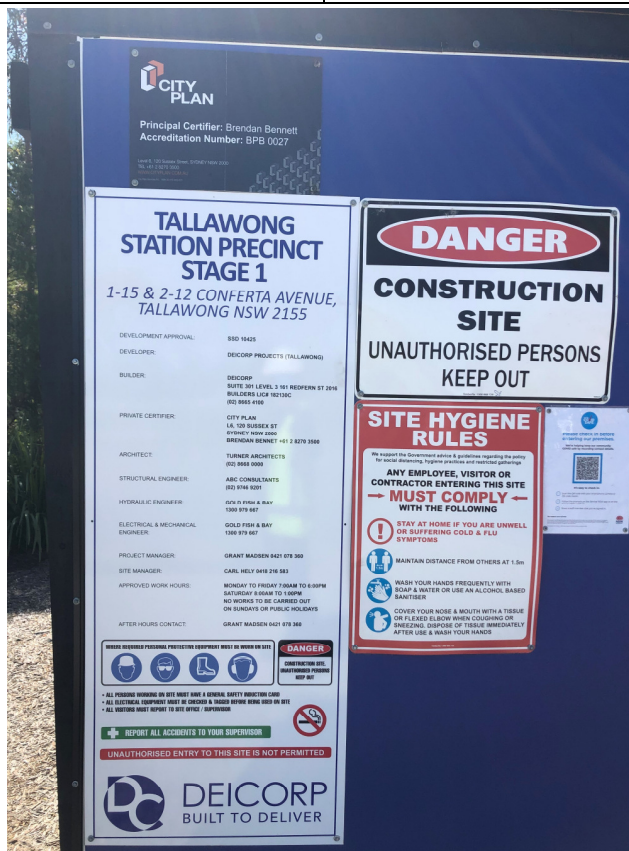
Photo 14: Site Notice compliant with Condition D2
