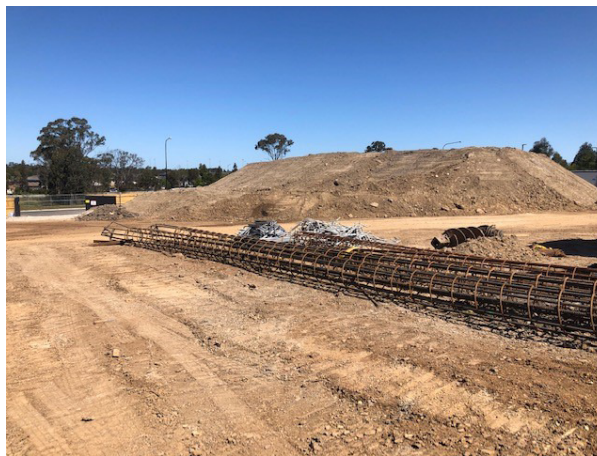
Photo 11: One of the two main stockpiles on site. The stockpile was being tested and classified prior to transport offsite.
